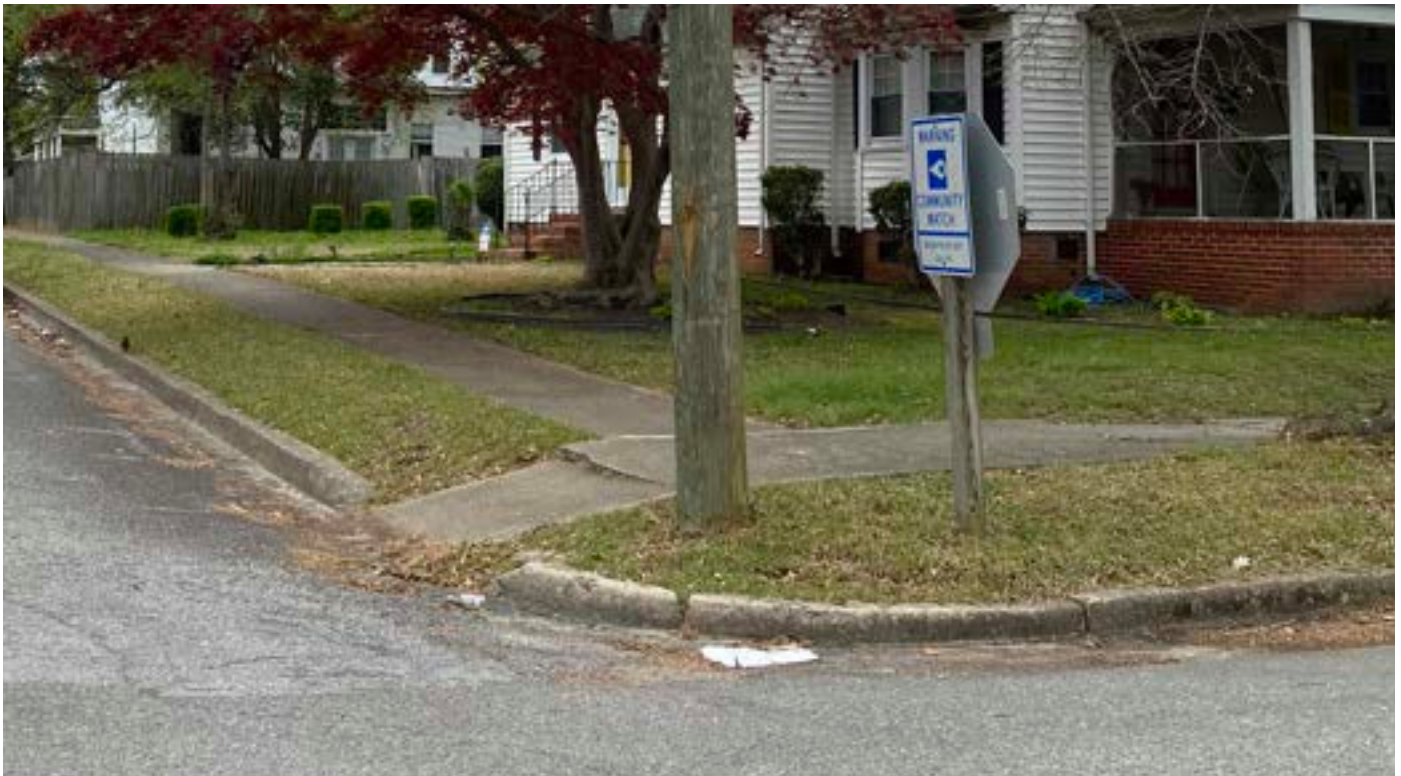
A non-ADA compliant curb ramp in Weldon
